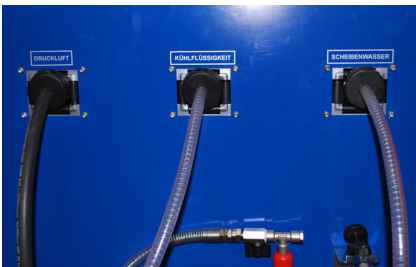
Built in hose reels
